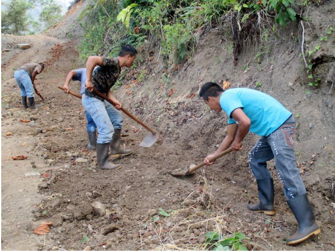
Lote 9 community members dig roadside ditches to prepare for the rainy season. No one else maintains the bumpy rock and dirt access roads. Photo by Sandra Cuffe for Mongabay.
