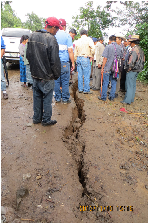
Large fissures have regularly opened in throughout San Miguel Ixtahuacan and Sipakapa, due to use of explosives in over 150kilometers of tunnels.
