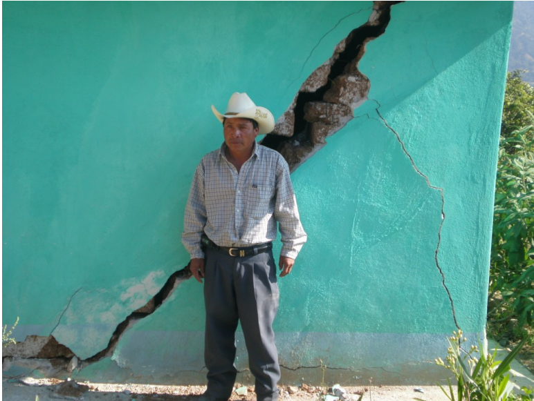
(Cracked house, community of Salitre, 2008. Photo @ Grahame Russell.)
